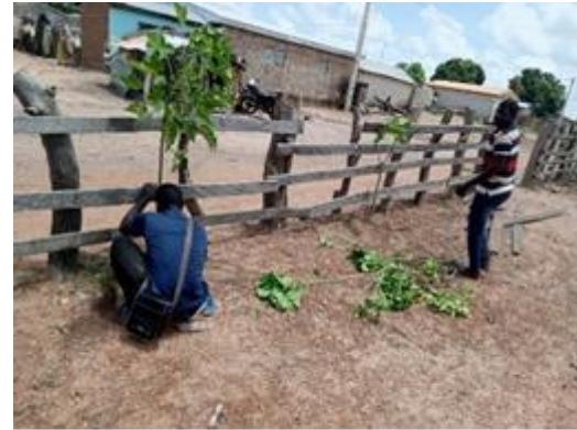
Goueya GAC building a fence around the Cultural and Education Action Center
